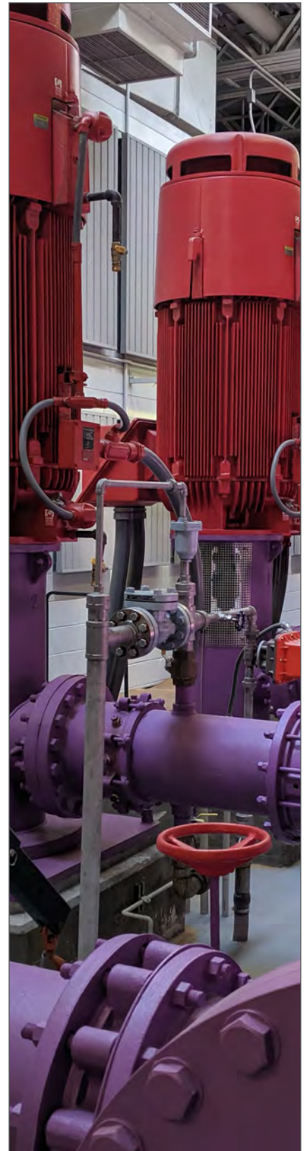
Reclaim Water System
