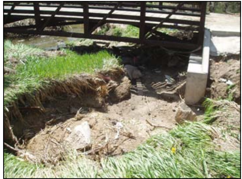
P4270015—Exposed Pedestrian Bridge Footer
