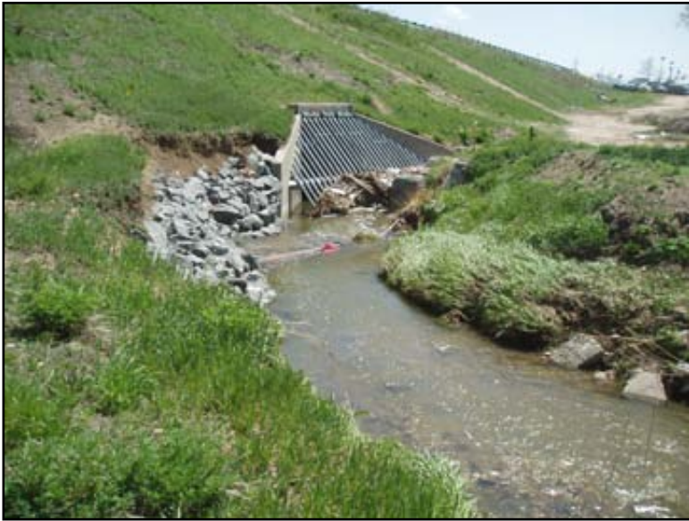
P4270011—Undersized Federal Blvd. Crossing w/ Exposed Sanitary Sewer
