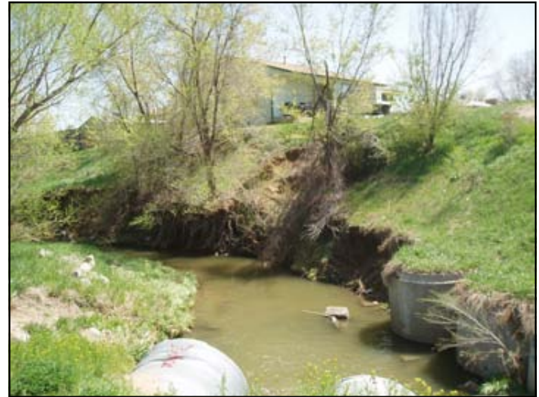
P4270021—Erosion d/s from 69th Ave Crossing
