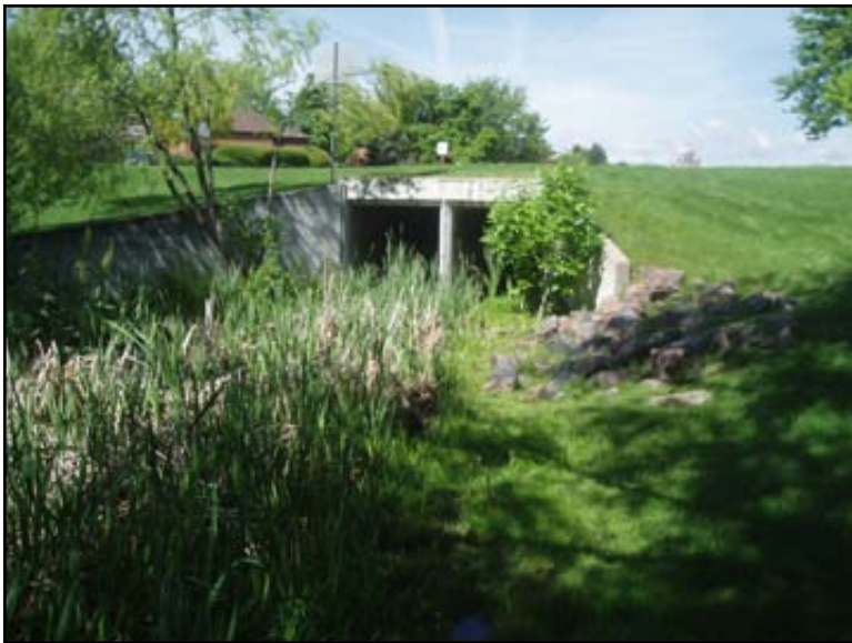
P5240009—Undersized (2) 6'x6' CBC Culvert at Quizas St.
