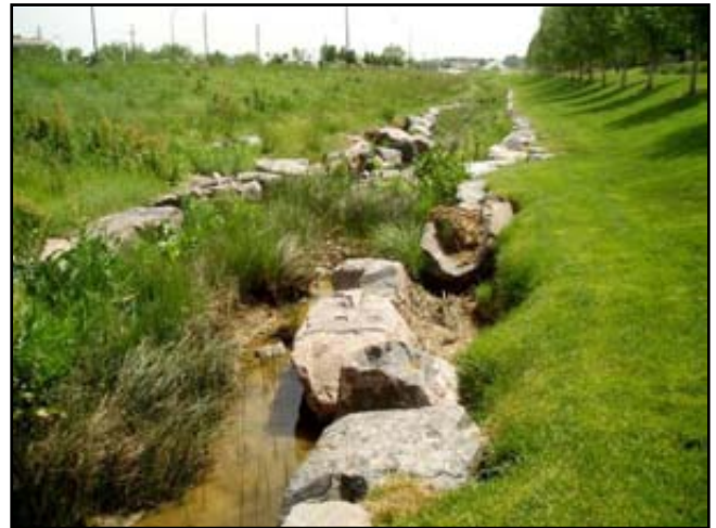
Failing Boulder Retaining Wall – City Park Drainageway
