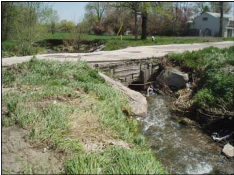
P4270016—Undersized Low Flow Street Crossing—Irving St.
