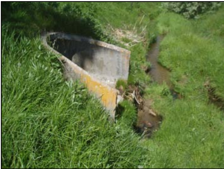
P5240013—Flared End Section Separating from Pipe
