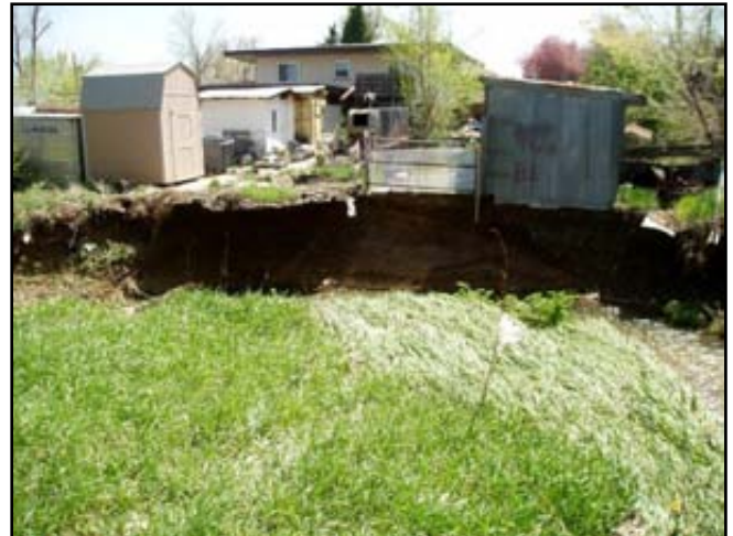
Severe Erosion – Little Dry Creek
