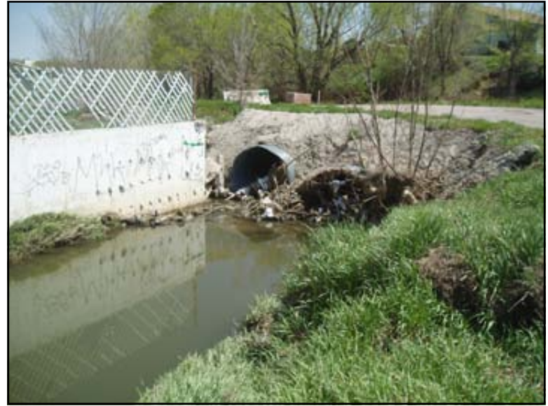
P4270023—Undersized 69th Ave Crossing
