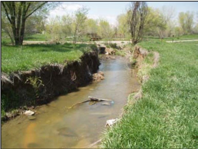
P4270013—Typ. Channel w/ Exposed Sanitary Sewer
