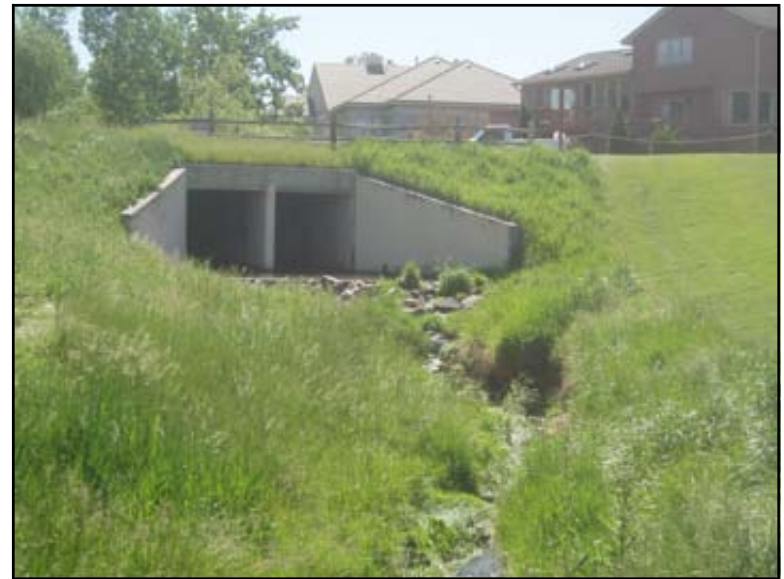
P5240010—Minor Erosion d/s of Quizas St. Outlet
