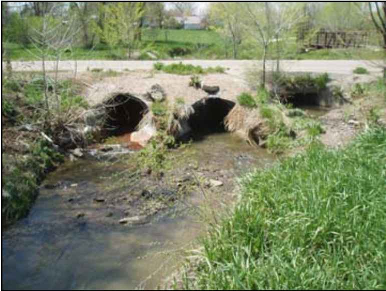
P4270014—Undersized Low Flow Street Crossing
