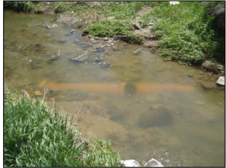
P4270012—Exposed Sanitary Sewer
